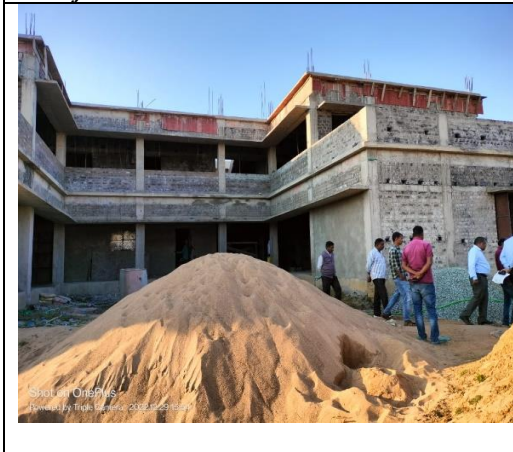
Image 5.2 : Incomplete Primary School Building at the Angulia R&R Colony, relating to the Kanpur Irrigation Project, Keonjhar
