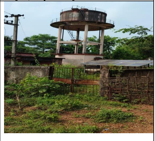
Image 5.3: Defunct Piped Water Supply System at the Rangamatia R&R Colony, relating to Subarnarekha Irrigation Project, Mayurbhanj
