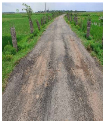
Picture 2.13.4: Depressed and damaged portions of BT road surface of BC road to Chhatrapada, in RW-II Bhadrak
