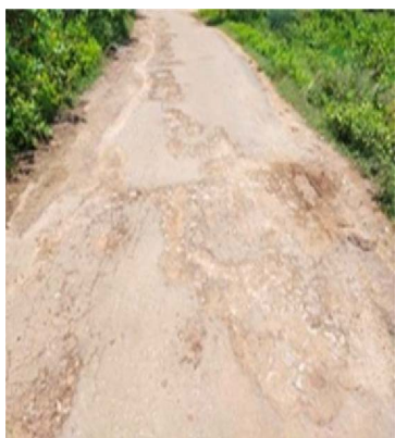
Picture 2.13.3: Crust failure and damaged surface of the PWD Road at P. Jagannathpur to Sunaripalli, in RW-II Ganjam
