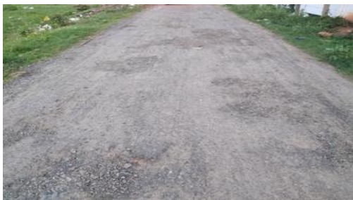
Picture 2.13.1: Damaged surface of NH-16, in front of the Golanthara Police Station to Gadakanallah road (RW Division-II, Ganjam), in the absence of three years’ post-construction maintenance
