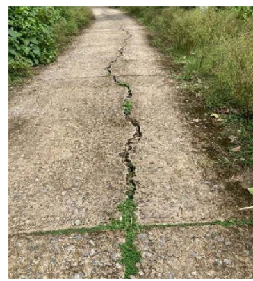
Picture 2.13.5: Cracks visible on the surface of the CC road in Barunasingh to Uttarachaka road, of RW-I Balasore
