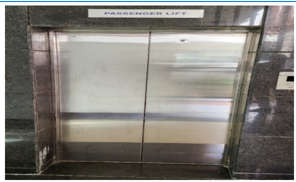
Picture 11.13 Elevators not in use due to non-maintenance (Tirupati Campus)
