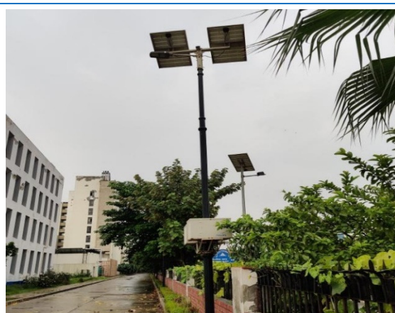
Picture 11.20 Defunct Solar Street Lights (Noida Campus)
