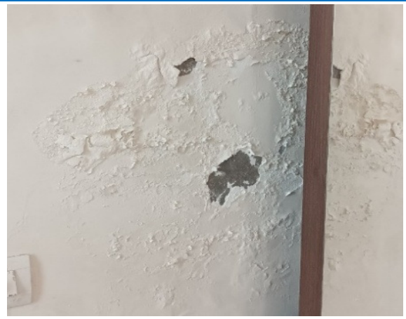
Picture 11.9 Dampness in the walls of Boys' Hostel (Tirupati Campus)
