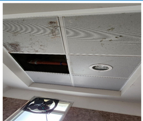
Picture 11.11 Washroom with missing tile in false ceiling (Tirupati Campus)
