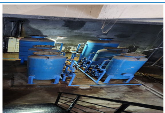
Picture 11.17 Non-functional Water Treatment Plant (Tirupati Campus)
