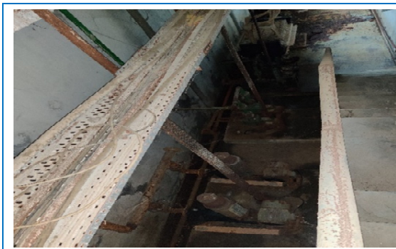
Picture 11.14 Non-functional Sewage Treatment Plant (Noida Campus)
