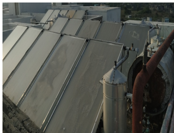
Picture 11.19 Non-functional Solar Panels on roof of Girls Hostel (Tirupati Campus)
