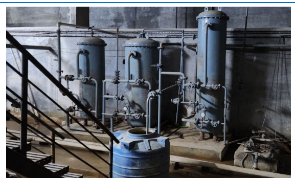
Picture 11.15 Non-functional Sewage Treatment Plant (Tirupati Campus)
