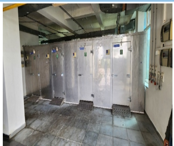
Picture 11.26 Unused walk-in freezers (Tirupati Campus)
