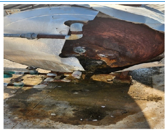
Picture 11.21 Damaged solar water heater (Tirupati Campus)
