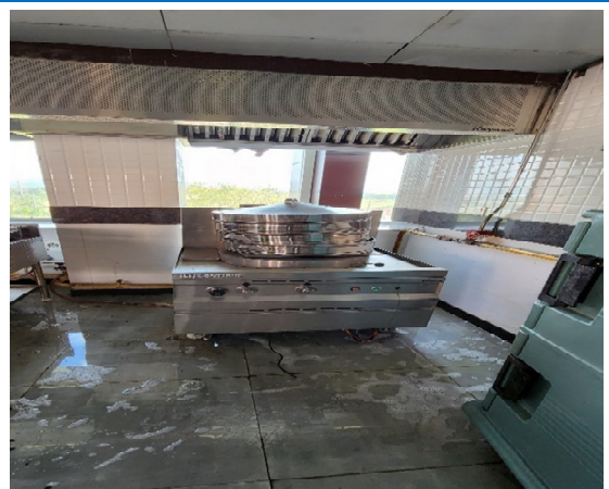
Picture 11.28 Unused Kitchen equipment in International Restaurant (Tirupati Campus)
