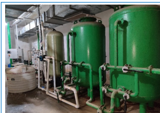
Picture 11.16 Non-functional Water Treatment Plant (Noida Campus)
