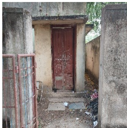
Mortuary Room in dilapidated condition at TH Kalaghatagi
