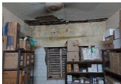
Dilapidated condition of the storage areas of TH Kalaghatagi.
