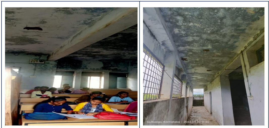
Students accommodated in dilapidated roof of building belonging to PU Education
