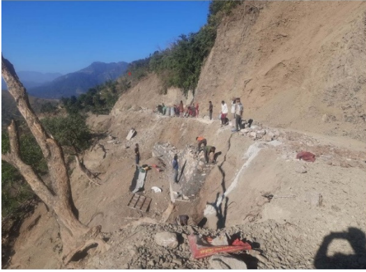
Workers working without safety equipment
