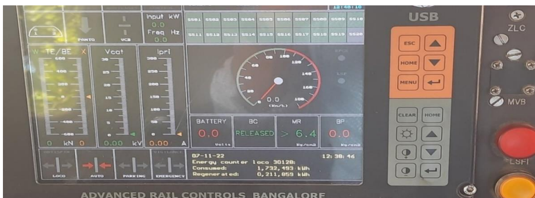
Image 1: Locomotive metering panel showing energy consumed and regenerated
