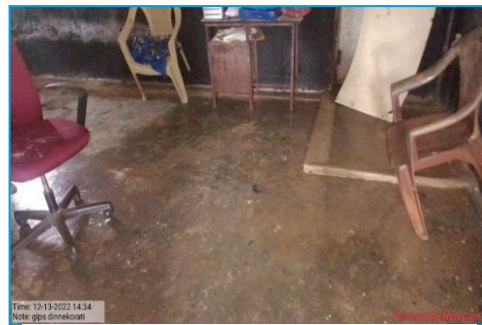
Condition of floor in GHPS, Dinnerakote, Bengaluru Rural
