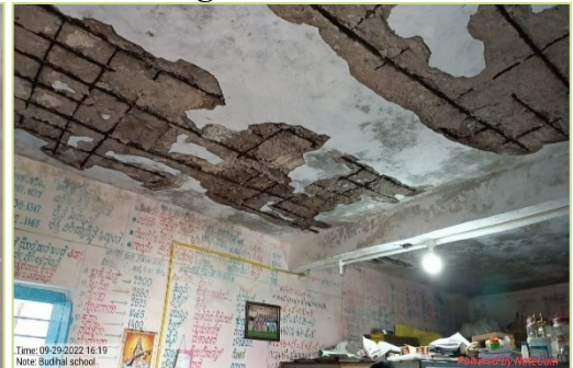
Condition of roof in GHPS, Budihal, Bagalakote
