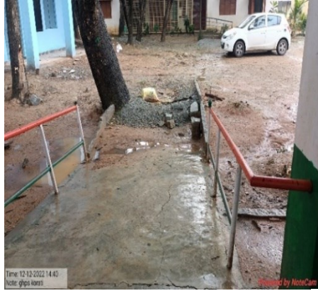
Inaccessible ramp GHPS Korati
