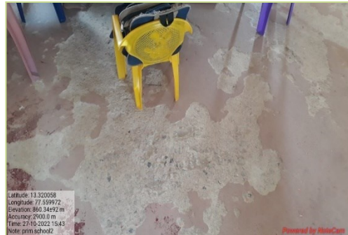
Condition of floor in GLPS, Thimsandra, Doddaballapura
