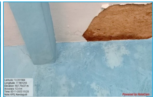
Condition of roof in KPS, Nandagudi, Hoskote
