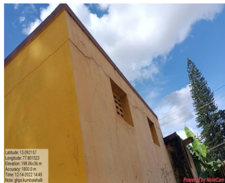
Poor construction of roof in GHPS, Kumbanahalli
