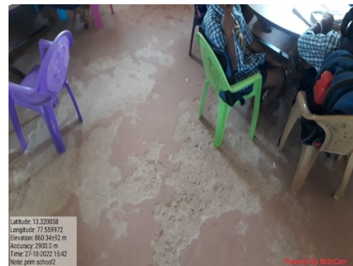
Poor construction of floor in LPS, Thimmasandra
