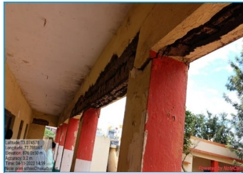
Condition of building in GHPS, Kuruburpete, Hoskote
