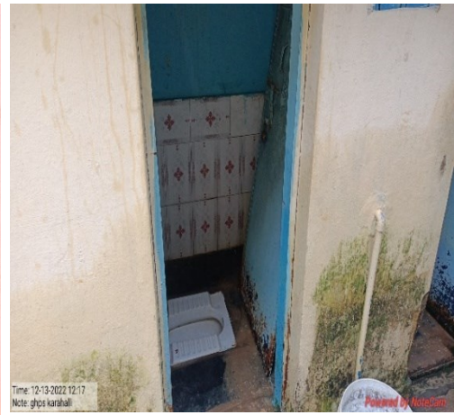
Toilet with broken door in GLPS Karahalli
