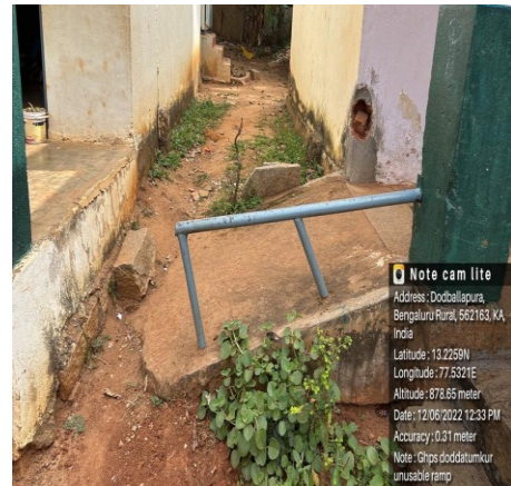
Unusable ramp in GHPS, Doddatumkur
