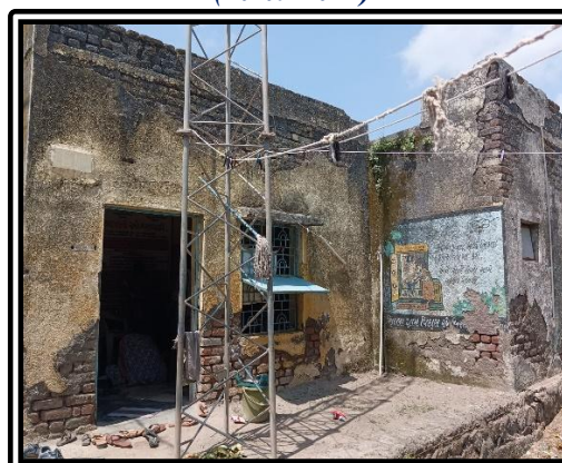
Picture 3.4: Dilapidated building of an AWC AWC: Barwala, Jasdan, Rajkot (Rural) (19-09-2024)
