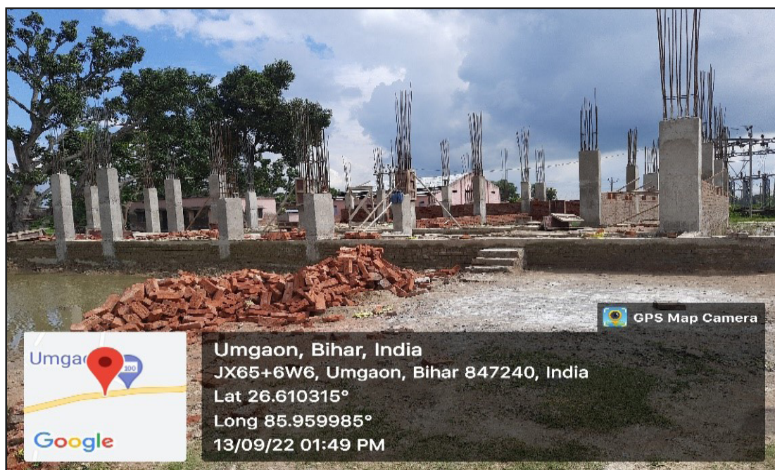
Image 5.2: Incomplete building of auditorium in Harlakhi, Madhubani
