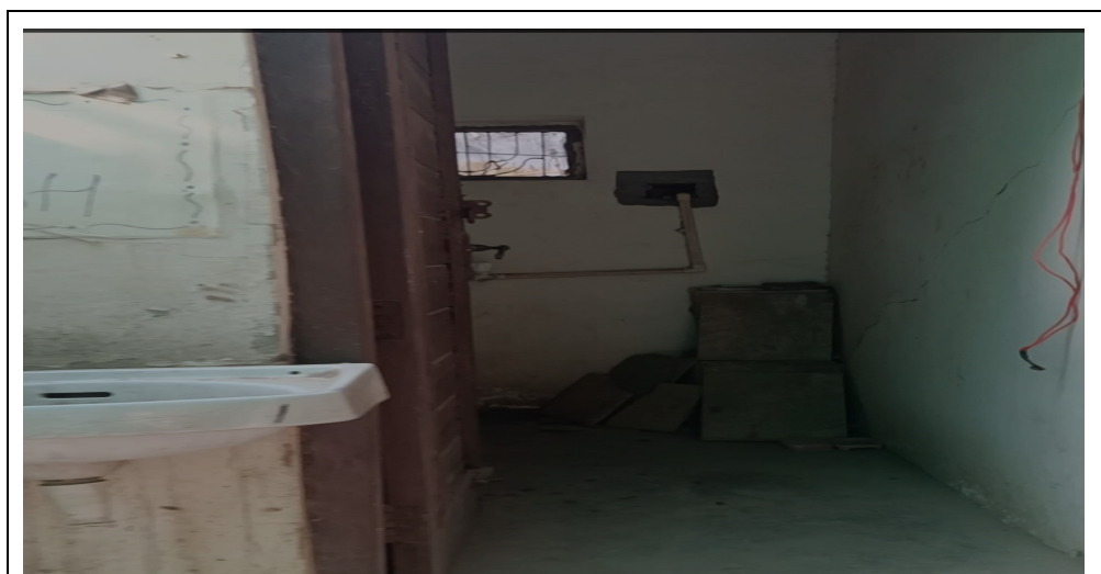
Picture-2.2.3: Toilet not functional
