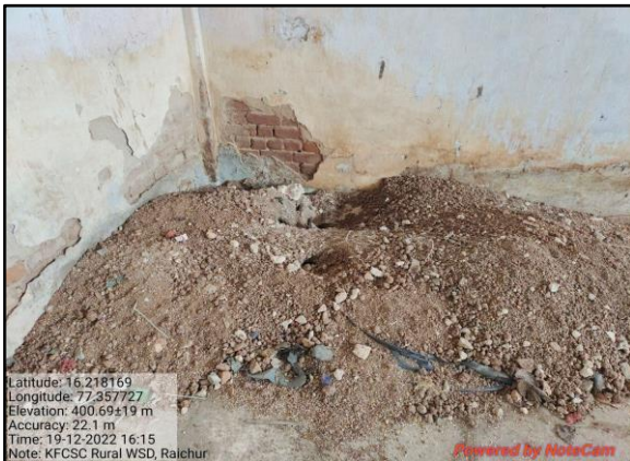
Rat burrows with dug-out mud were found in the corner of the GTF WSD - KFCSC Raichur.
