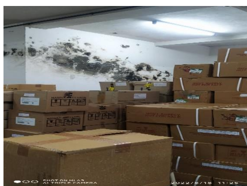
Photo 4.3: Drugs stored adjacent to damp walls.
