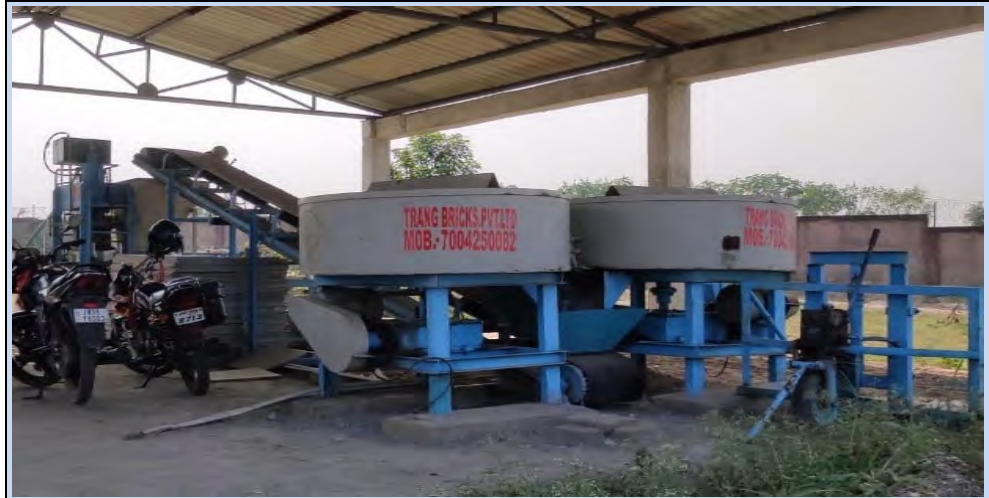
Exhibit 9.7: Non-functional brick making plant at the Deoghar Municipal Corporation (photograph taken on 12 November 2022)
