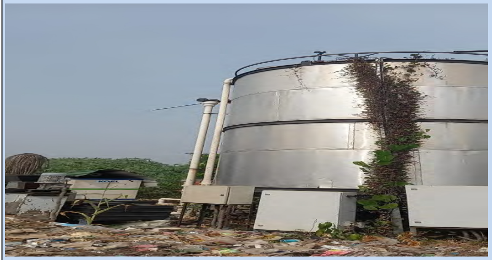
Exhibit 9.9: Idle bio-methanation plant at the Deoghar Municipal Corporation (photograph taken on 12 November 2022)
