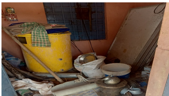
Picture-5: Defunct treatment unit and pump house at Bambilo village
