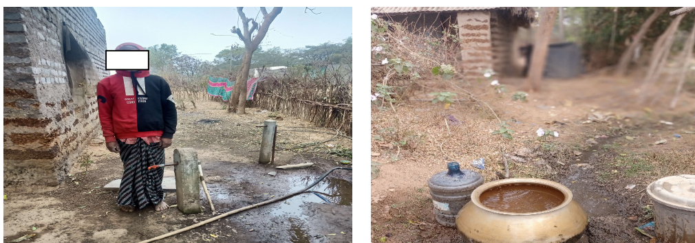
Picture- 3 and 4: Leakage and broken tap of the households at Mithigaon Village of Hatadihi block
