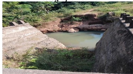
Collapsed Box Cell Bridge at Sunki GP of Pottangi PS
