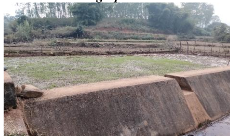
Check dam at Khajuriput of the Goudaguda GP of Laxmipur PS, without any space for storage of water
