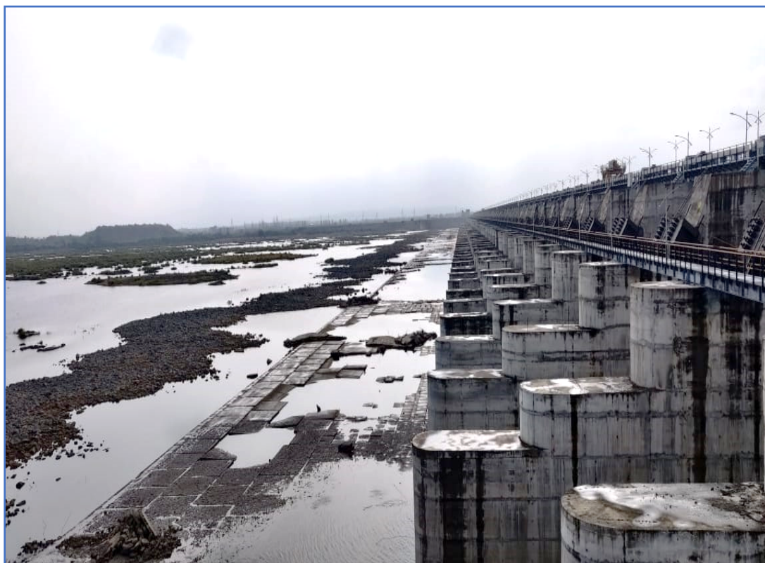
Figure 5.2 – Damaged CC Blocks and apron at downstream side of Sundilla barrage
