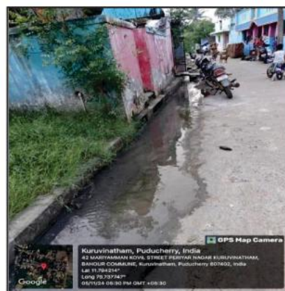
Picture 2.9: Stagnation of water on streets due to absence of greywater management
