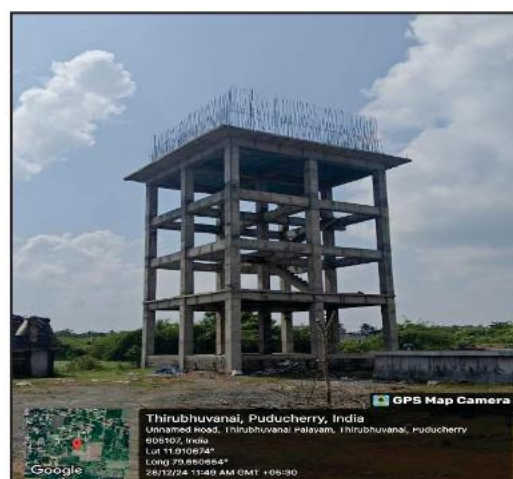
Picture 2.12: No progress in the work at Thirubhuvanaipalayam and rods exposed to open air
