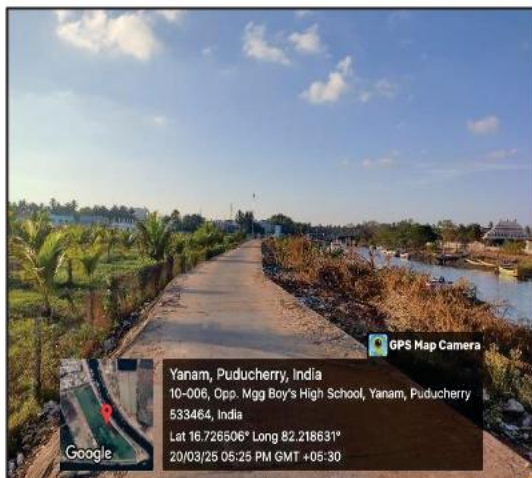
Picture 2.17: Unfinished work (pathway laid without provision of facilities)
