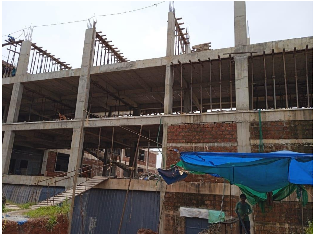
Figure 5.6: M/s Hillsinai building, Markaz Knowledge City, Kaithappoyil, Kozhikode. Failure to provide safety net of standard. Photo taken by Audit party on 21 September 2023.
