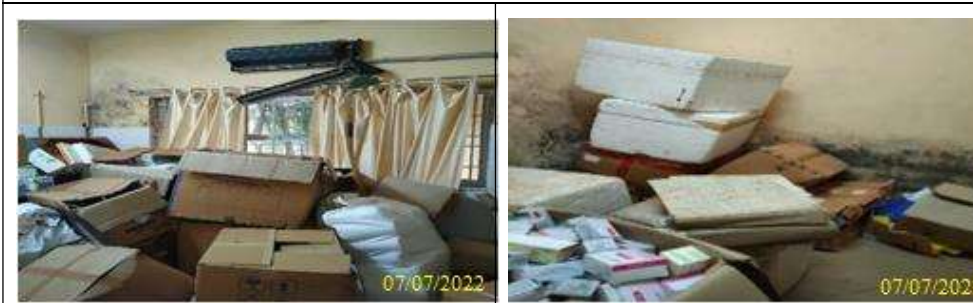
Photo No.4.7 and Photo 4.8: Medicines boxes dumped on floor, soiled walls in drugs stores room. (CHC, Canacona)
