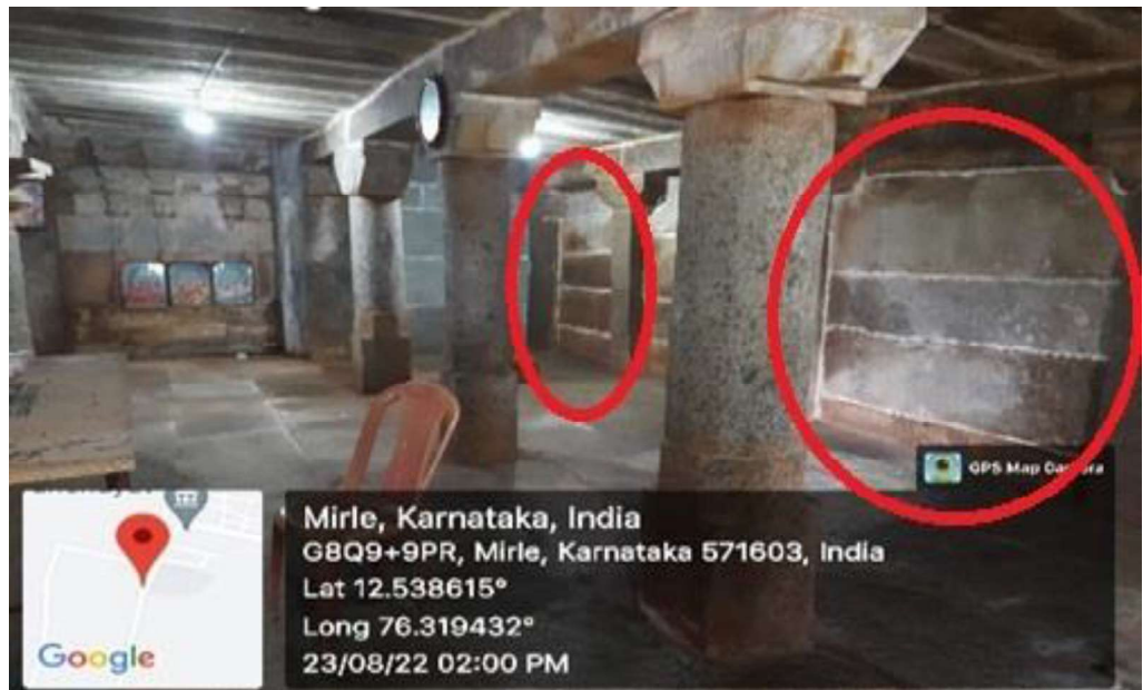
Picture No 4.24: Cement used for filling joints at Sri Yoganarasimha Swamy Temple, Mirle, K R Nagar Taluk.
