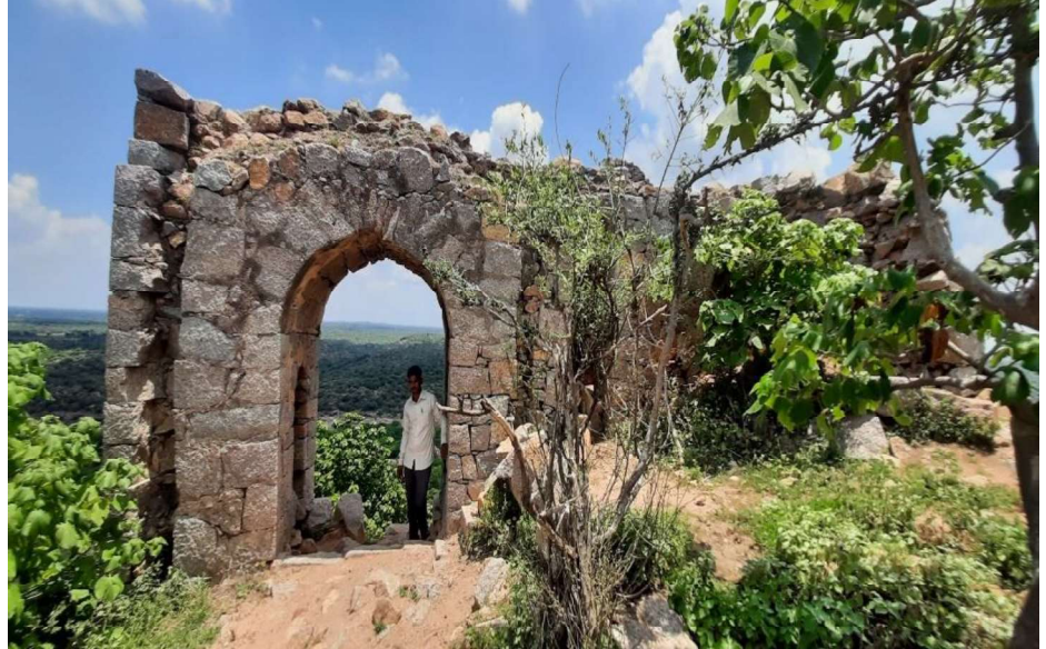
Picture No. 4.3: Non-prioritisation of conservation work at Jaladurga Fort, Lingasugur Taluk, Raichur District.
