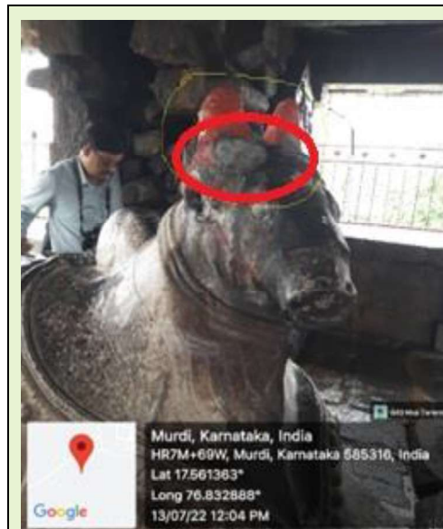
Picture No 4.26: Cement used in repairing the damaged Nandi Idol at Sri Ramalingeshwara Temple, Hodal, Kalaburagi District.
