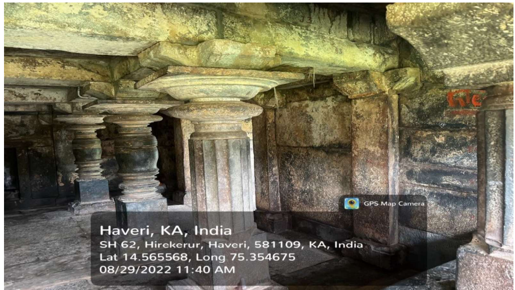
Picture No 4.45: Condition of Ishwara Temple at Hansabhavi, Hirekerur Taluk, Haveri District due to seepage of water and growth of algae.
