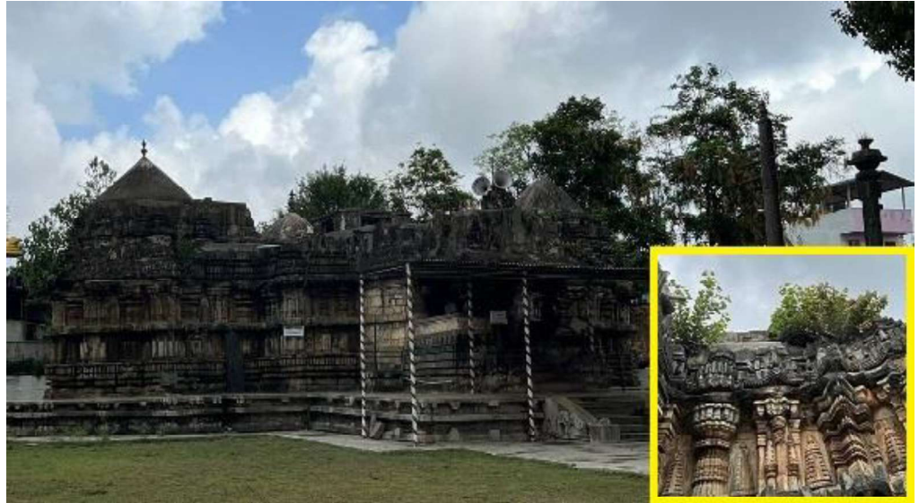
Picture No 4.19: Growth of Peepal Tree and algae on monument notified during 1930 at Sri Lakshminarasimha Swamy Temple at Bhadravathi Taluk, Shimoga District (Non sample).
