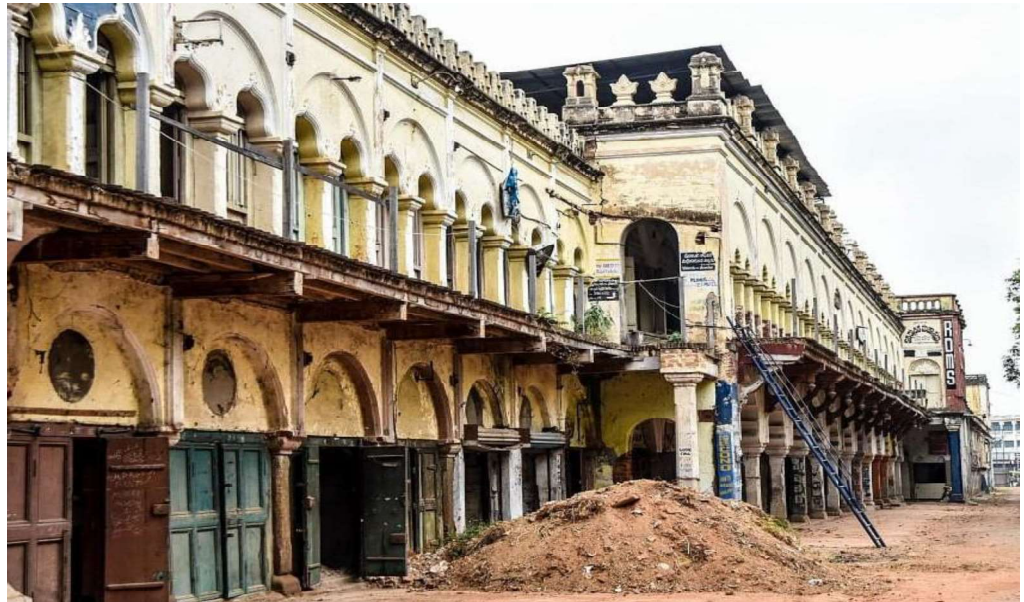
Picture No. 3.16: Crumbling Lansdown Building identified as a heritage monument at Mysuru.
