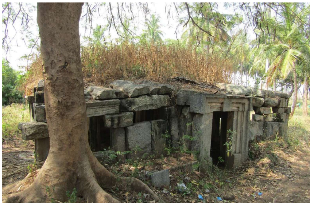
Picture No. 3.2: Damaged monument identified during survey at T Narsipura Taluk, Mysuru District.
