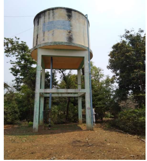
Exhibit 3.2: Chlorination unit installed in an OHT
