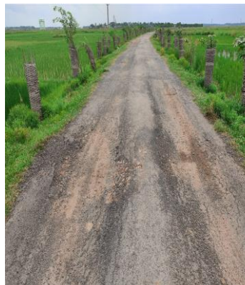
Picture 2.13.4: Depressed and damaged portions of BT road surface of BC road to Chhatrapada, in RW-II Bhadrak
