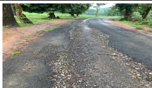
Picture 2.13.2: Guliguda road, RW Division, Jeypore, in the absence of first years' maintenance
