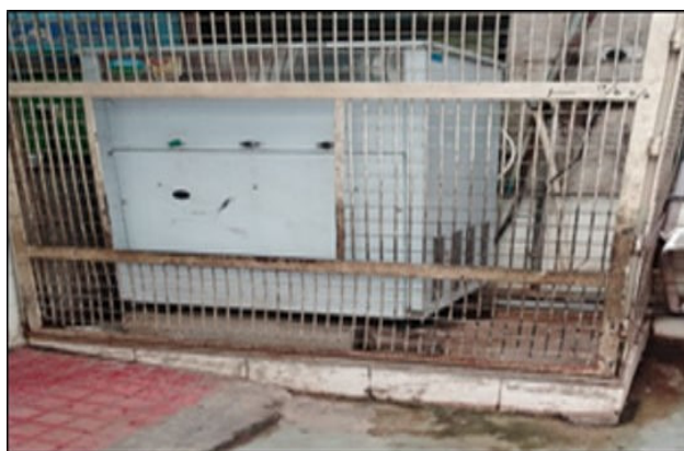
Picture 3.3: Water cooler not functioning in CNBC
