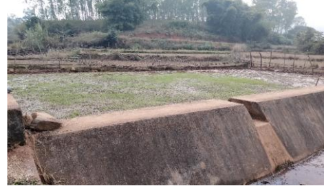
Check dam at Khajuriput of the Goudaguda GP of Laxmipur PS, without any space for storage of water
