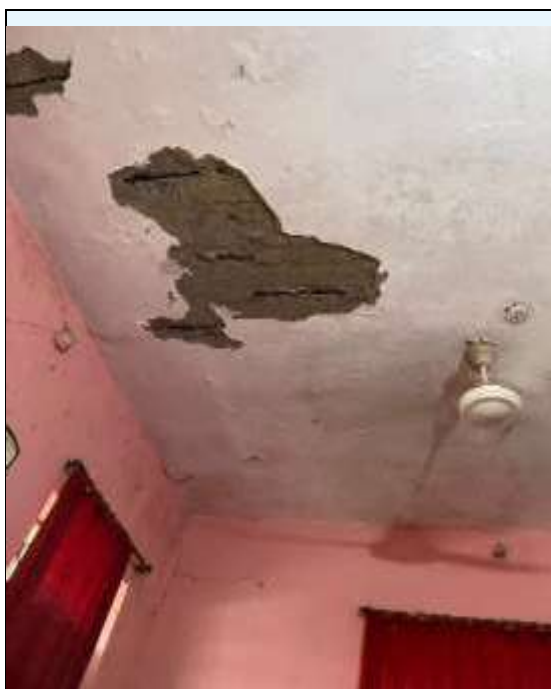
34. Dilapidated ceiling at GAD, Namnakala (Surguja) (31 March 2022)
