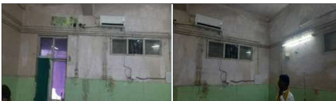
13. Dilapidated condition and seepage in burn ward in GMCH Bilaspur (Date 20 April 2022)
