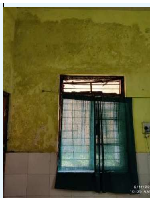
35. Seepage problem in DH, Jagdalpur (11 June 2022)
