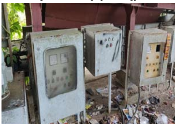
Exhibit 6.9: Damaged panel board of compost plant
