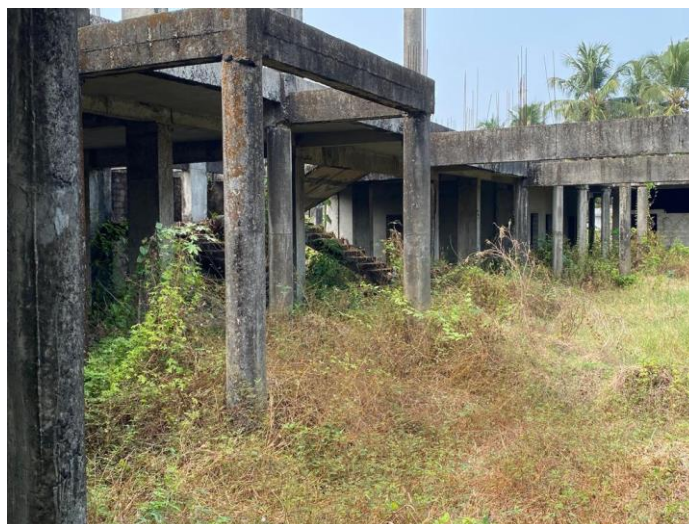
Figure 5.3: Abandoned building at Government Ayurveda Panchakarma Hospital, Alappuzha. Photograph taken on 16 February 2022
