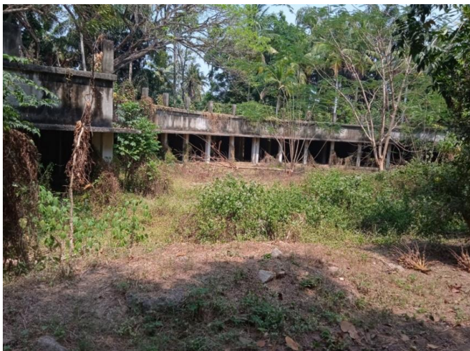
Figure 5.2: Abandoned Male Forensic Ward in GMHC, Thiruvananthapuram Photograph taken on 08 February 2022
