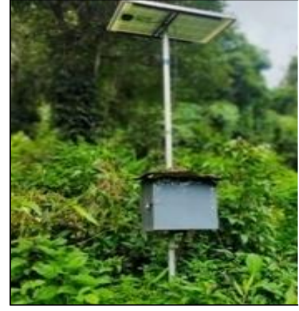
Figure 2.6: Non-functioning solar fence - Bimaram in Ranni range (23 September 2021)
