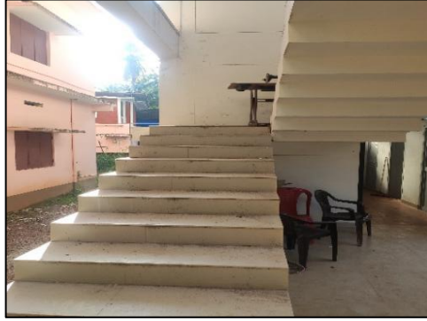
Figure 2.13: GHSS Parayanchery, Kozhikode - stair without handrails provided
