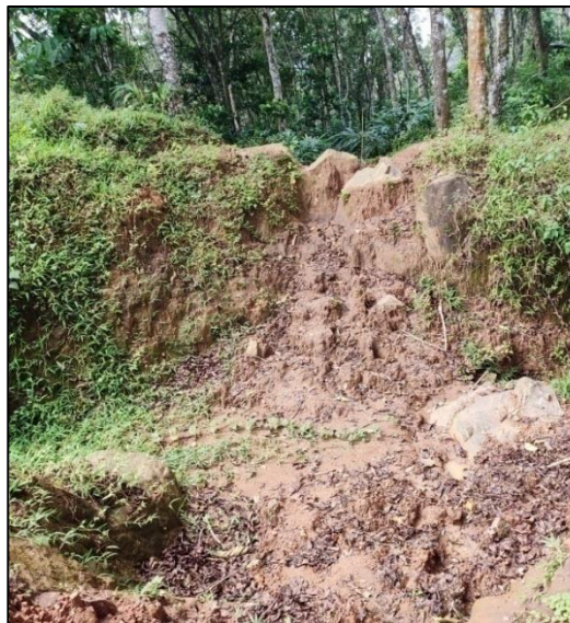
Figure 2.7: Damaged EPT - Periyar East Division (08 December 2021)
