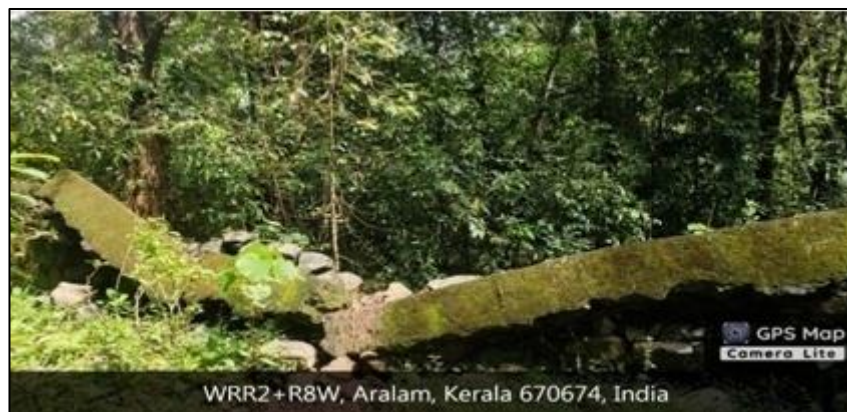
Figure 2.9: Damaged EPW- Aralam Wildlife Sanctuary (16 November 2021)
