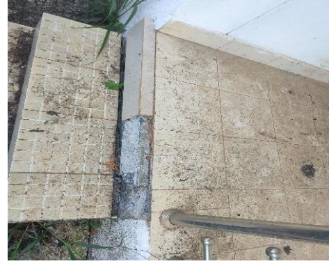
Figure 2.22: Cracked tiles in Ministerial Staff Quarters, Kozhikode
