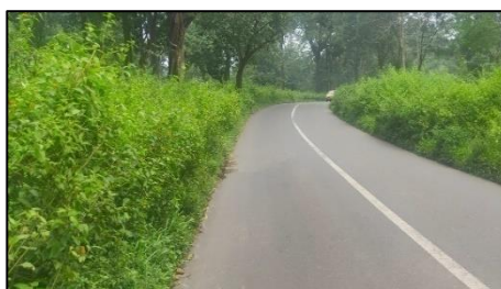
Figure 2.10: Vista clearance not done – Sulthan Bathery – Pulpally road under Wayanad wildlife division
