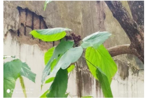
Figure 2.18: Exposed reinforcement at EC Block, CET, Thiruvananthapuram
