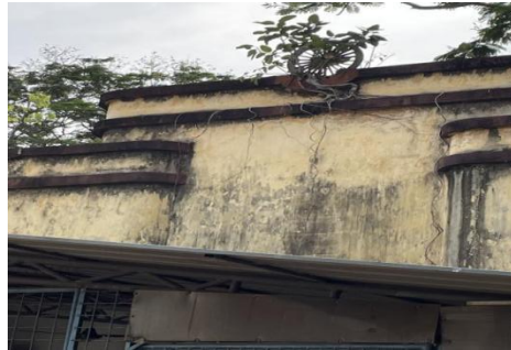
Figure 2.17: Vegetation growth on building at ITI, Chakkai, Thiruvananthapuram
