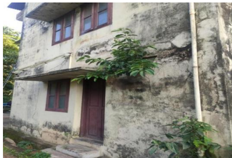
Figure 2.19: Cracks and vegetation growth in Pavamani Quarters, Kozhikode
