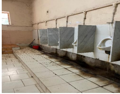
Figure 2.21: Badly maintained toilet at Civil Station, Thrissur
