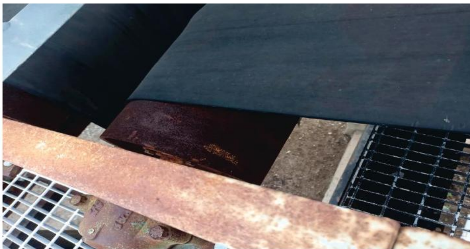
Pictures showing the rusted/damaged parts of 100 TPH washery
