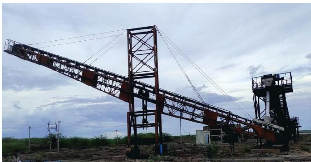
Picture showing the installed 100 TPH washery at site
