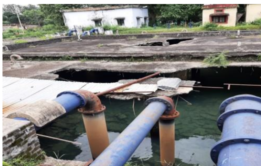
Sump well at RFP
