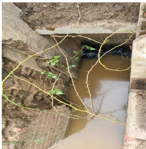
Regulator gate not installed at the head of Masoodpura minor of DCS
