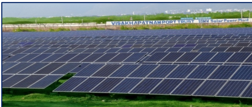
Picture 7.8 – 10 MW Solar Plant at VPA
