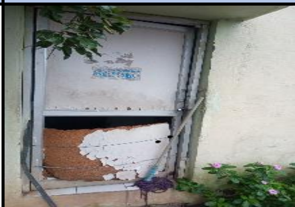
Figure 19: A closed toilet in a Truck Lay-bye located in Karur- Dindigul stretch (Chainage 304.100 km, LHS) - Velanchettiyur BOT Toll Plaza
