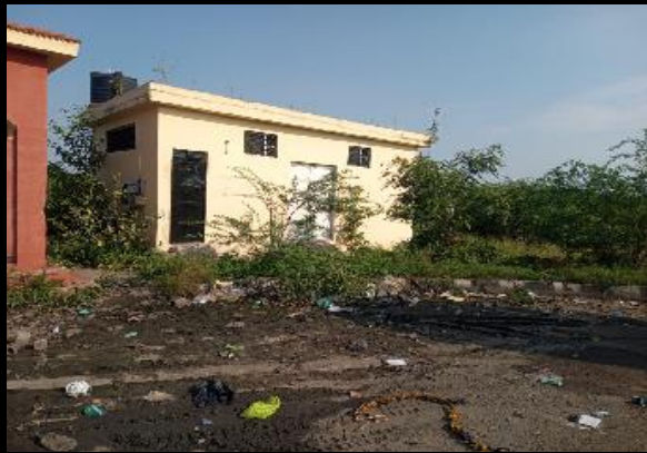
Figure 17: A toilet in the Truck Lay-bye located in Tambaram Tindivanam stretch in shabby & locked condition (Chainage 69.800 km, LHS) - Paranur Public Funded Toll Plaza
