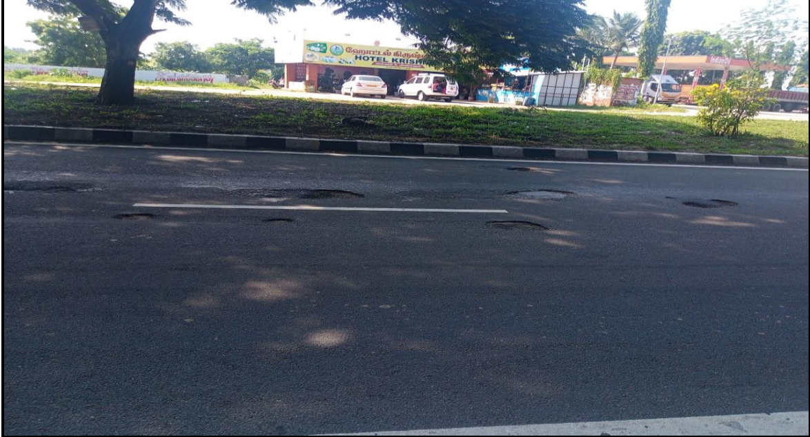
Figure 8: Picture of Potholes on Tambaram-Tindivanam stretch (NH 32) found during Joint Inspection
