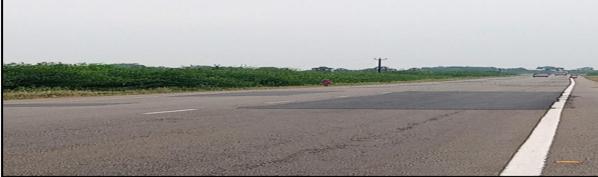
Figure 9: Picture showing uneven patches on Trichy-Karaikudi stretch (NH 36) found during Joint Inspection
