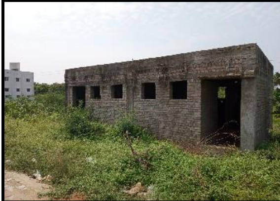
Figure 16: An incomplete structure in a Truck Lay-bye in Madurai Kanyakumari stretch (Chainage 11.200 km, RHS) - Kappalur Public Funded Toll Plaza
