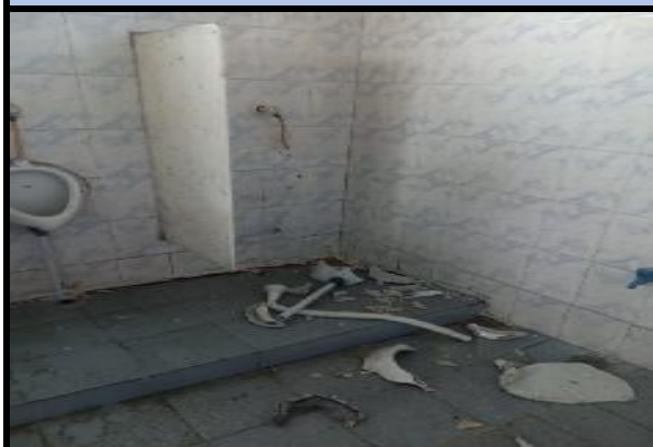
Figure 18: Inside view of a toilet in the Truck Lay-bye located in Tambaram Tindivanam stretch (Chainage 69.800 km, LHS) - Paranur Public Funded Toll Plaza
