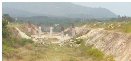
Incomplete structure on Feeder canal
