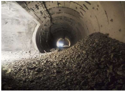
Excavation of Adit from Tunnel I to II for manual excavation in Tunnel II. Until closure of Adit, release of water through tunnel I is not possible
