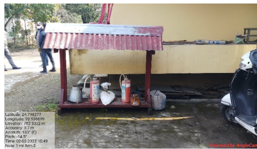
Sand buckets without sand and expired fire extinguishers (1 st Battalion Manipur Rifle)
