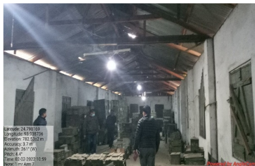
Storage of arms in the old barrack with water leakages (Arms KOTE at 1 st Battalion Manipur Rifles)
