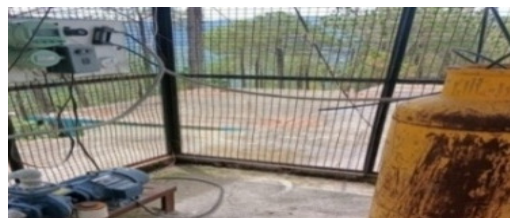
Gaseous chlorination plant
