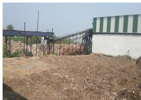
Incomplete solid waste treatment plant at Deoghar.
