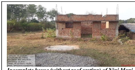
Incomplete house (without roof casting) of Nini Mani Harijan, ID No. OR4703427 of Kosagumuda GP/Block of Nabarangapur District, shown as completed in AwaasSoft, with payment of full assistance of ₹ 1.30 lakh.
