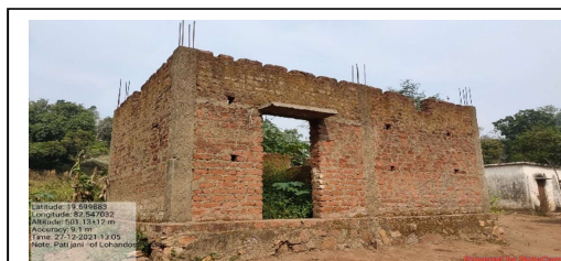
Incomplete house (without roof casting) of Pati Jani, ID No. OR4666180 of Chakalapadar GP of Jhorigam PS of Nabarangapur District, shown as completed in AwaasSoft, with payment of full assistance of ₹ 1.30 lakh.
