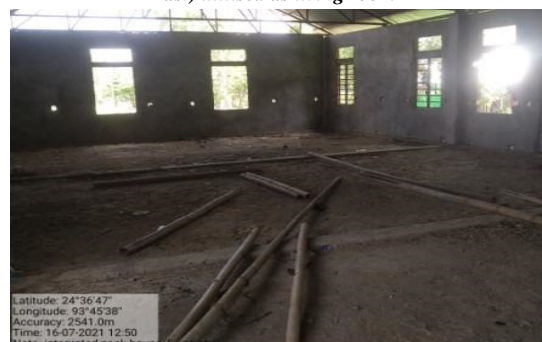
Incomplete Integrated Pack house of Integrated Rural Area Development Organisation (IRADO) at Kwasiphai, Bishnupur
