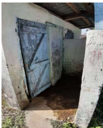
Dysfunctional toilet in Government upper primary school, Pukhuri
