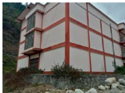
Building without 'Boundary Wall and Protection Wall'.
