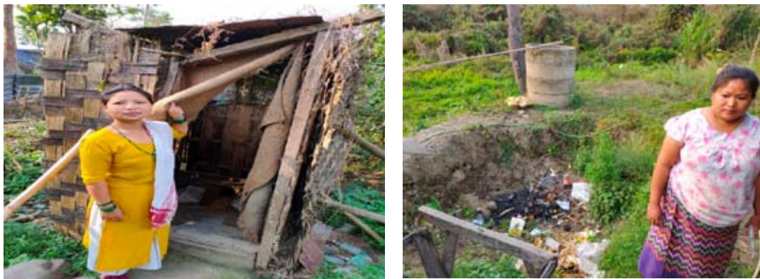
Insufficient supply of material resulted in construction of insanitary toilet
