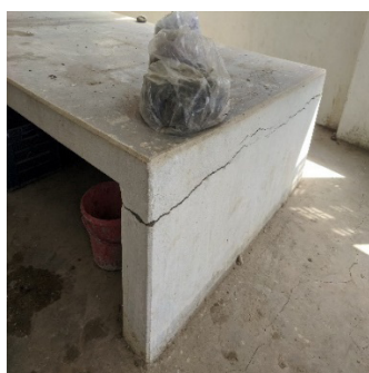
Cracks on elevated platform
