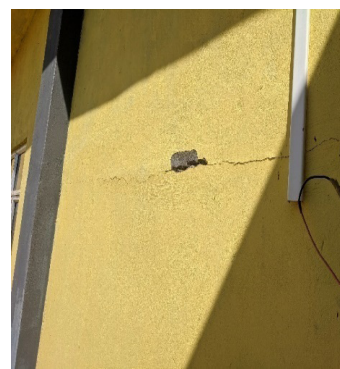
Cracks on outer wall
