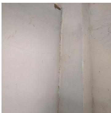
Cracks on partition wall
