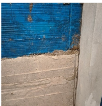
Cracks on ceiling of ground floor
