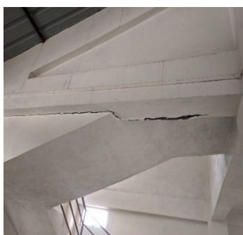
Cracks on ceiling and wall
