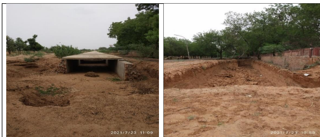
Images showing unutilised incomplete drain (23.07.2021)
