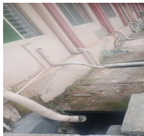
Kochi Corporation Palluruthy Taluk Hospital - Bio-medical liquid waste is let out directly to drainage (November 2021)
