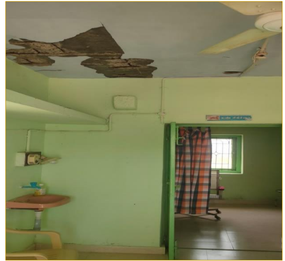
Exhibit 5.8: Damaged Roof at UPHC, Chennimalai
