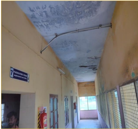
Exhibit 5.7: Water seepage at non-Taluk hospital, Thanipadi
