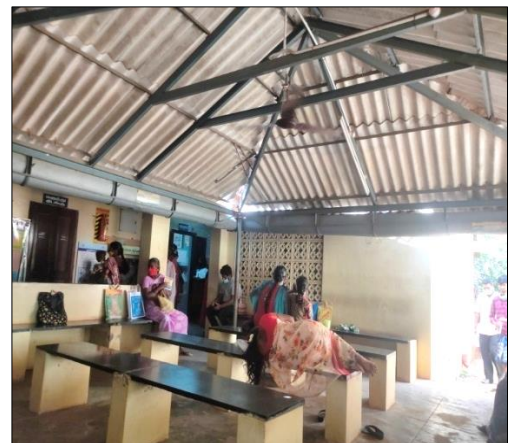
Exhibit 3.8: OP counter functioning under asbestos sheet at Urban PHC, Modakuruchi
