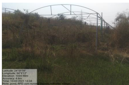
Completely damaged polyhouses (Ukhrul district)
