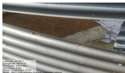
Damaged water tank at Thawai Farm
