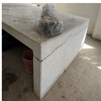
Cracks on elevated platform
