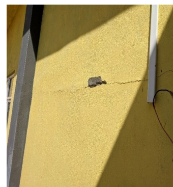
Cracks on outer wall
