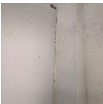
Cracks on partition wall
