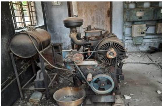
Picture 5.5: Non-functional generator at Hingalganj PHC, Bashirhat (April 2022)
